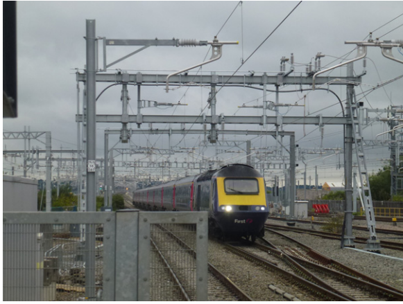
Fig. 1. Great Western electrification project OLE infrastructure at Reading
